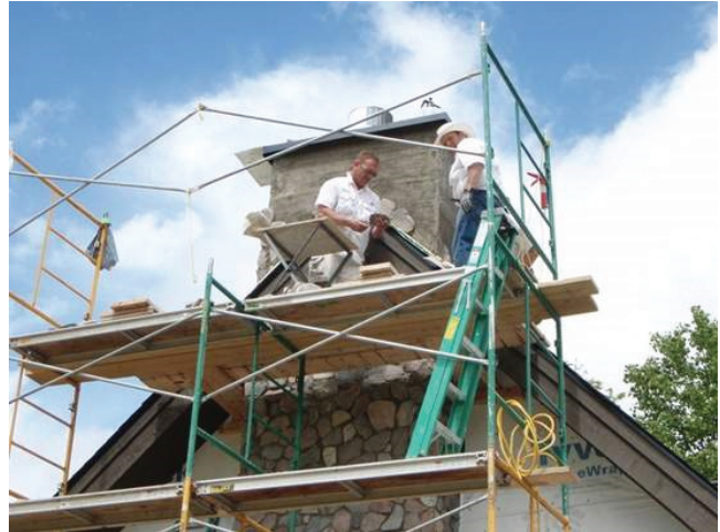
Jason Buechel, left, and his uncle, Dave Patoka, add stone to a chimney on the Believe in Tomorrow House at Pinnacle Falls in Zirconia, N.C. (Submitted photo)
